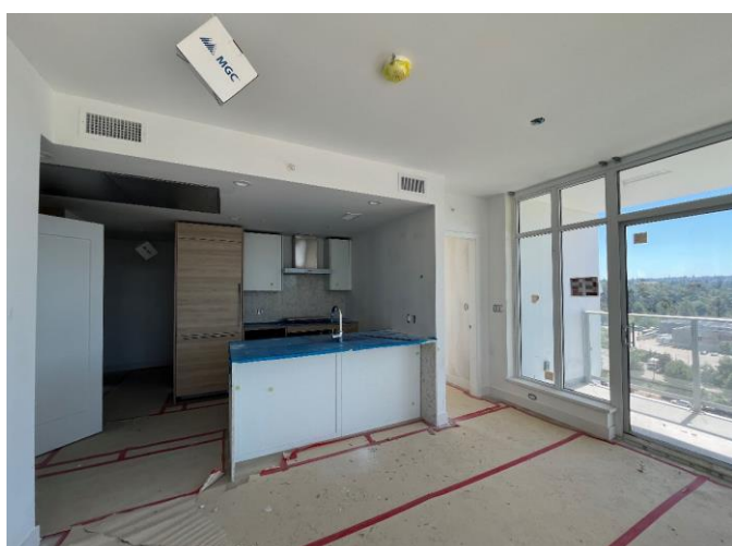
L10 - Appliance installed
